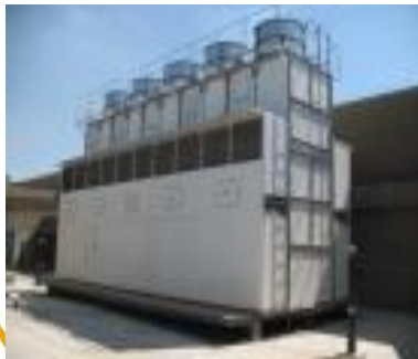
Indirect evaporative chiller
