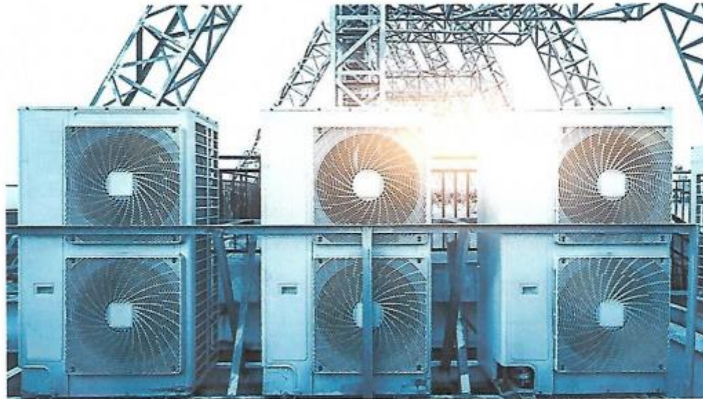
Efficiency improvements could cut the energy growth from air conditioner demand in half through mandatory energy performance standards (Photograph: Getty Images)
